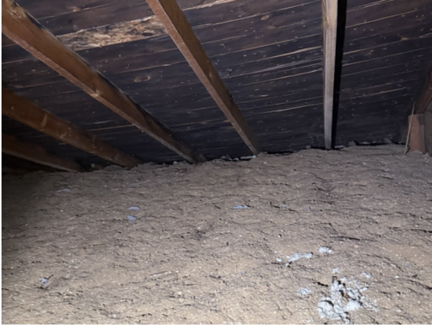
The black mold will be mitigated by a new ventilation system, which will allow the new shingles to have their maximum life.
